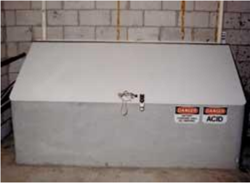
Air-tight insulated battery box with PVC air vents to the outside
