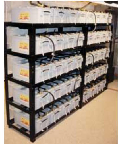
Rack-mounted solar gel-cell sealed batteries
